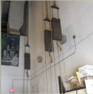
SMS GLE, MBE, CES Replace Stage Rigging and Lighting (ACM wiring) CMPL
